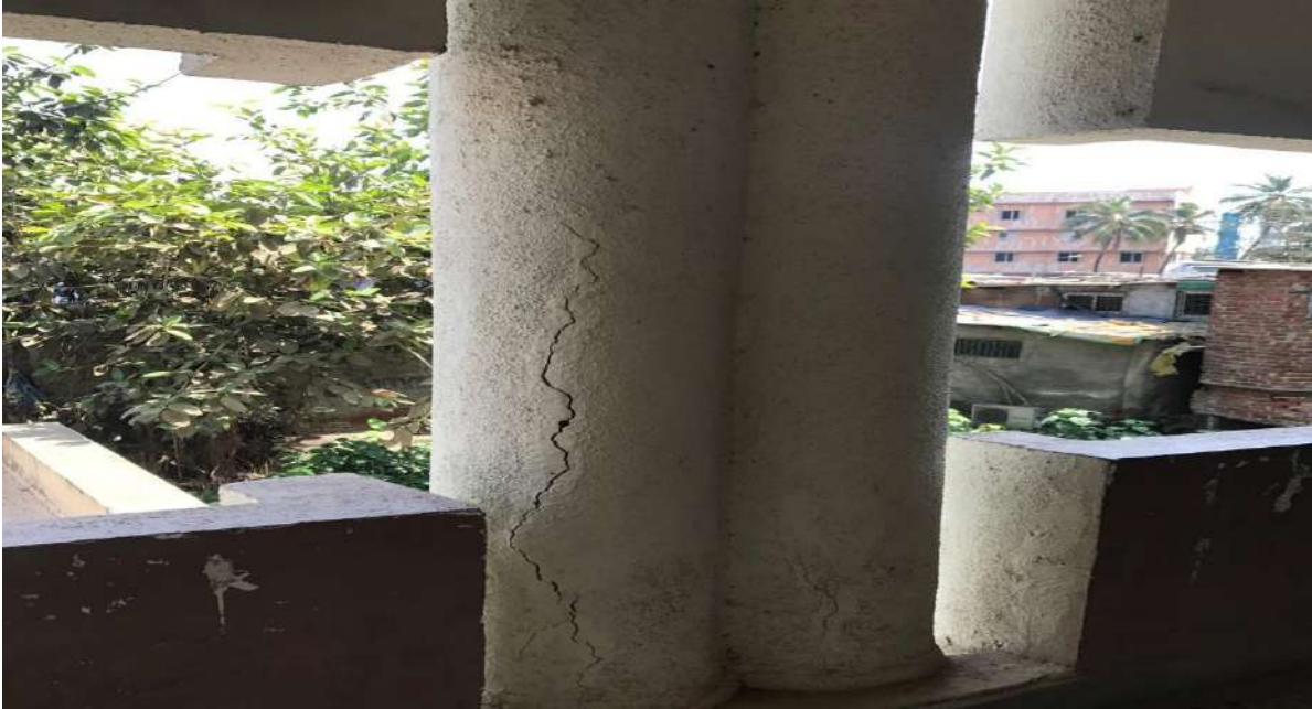
PH NO-42:-Photograph showing crack on column at various locations of passage.
