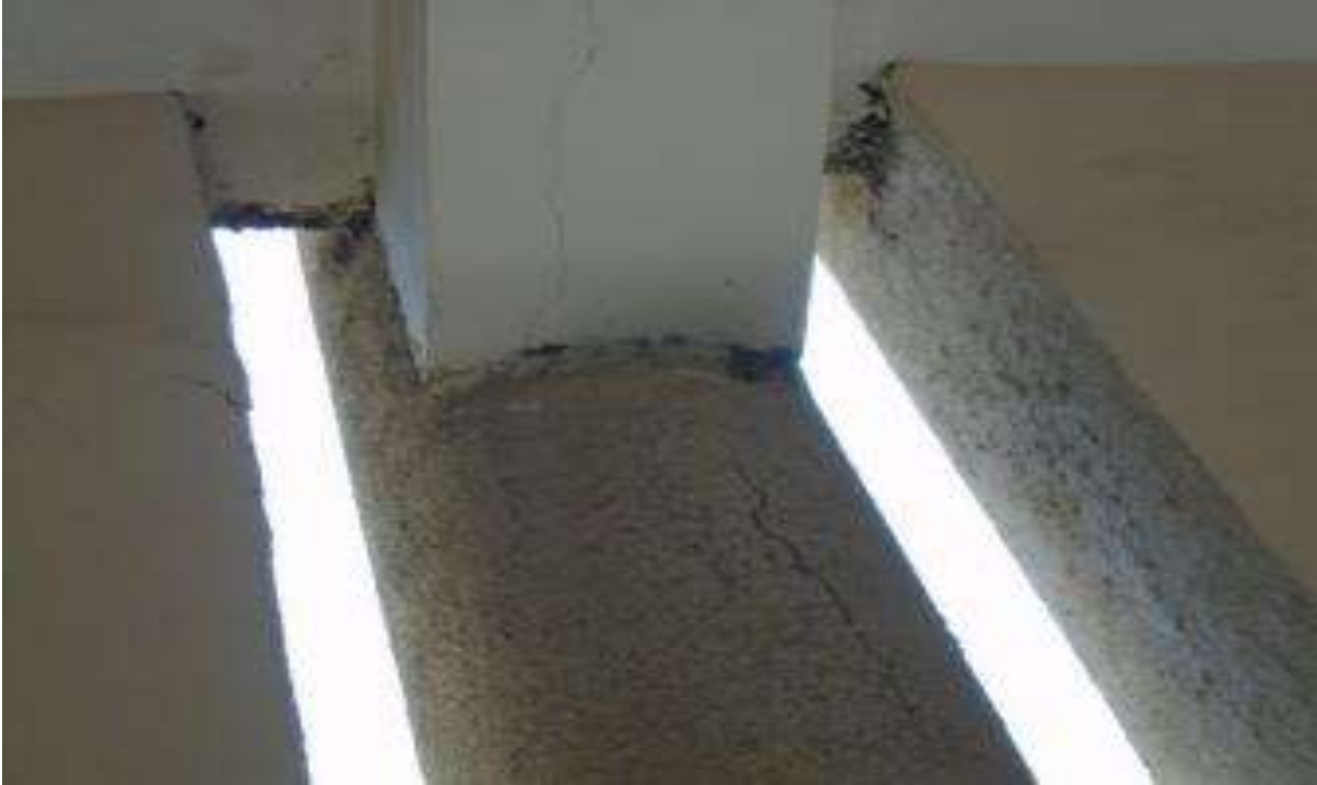
PH NO-25:-Photograph showing crack on column and beam at passage.
