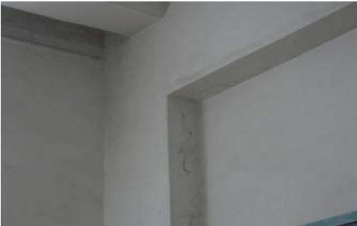
PH NO-11:-Photograph showing crack on column at office no- 24.
