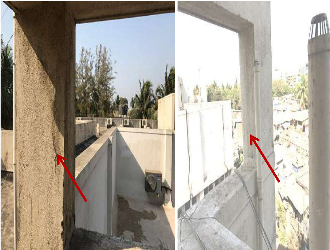
PH NO-24 & 25:-Photograph showing crack on column overhead tank.
