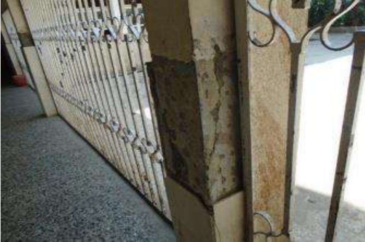
PH NO-31:-Photograph showing crack on column at passage.
