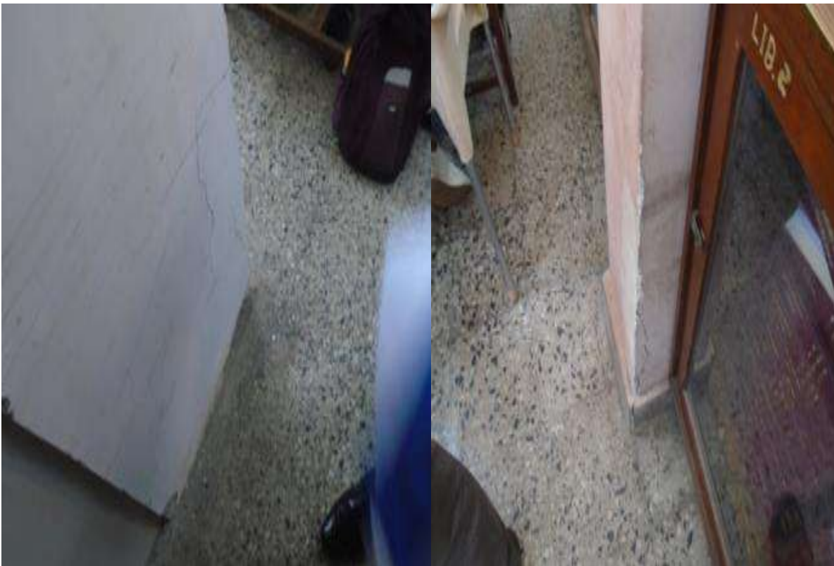
PH NO-03 & 04:-Photograph showing crack on column bottom at office no-27.
