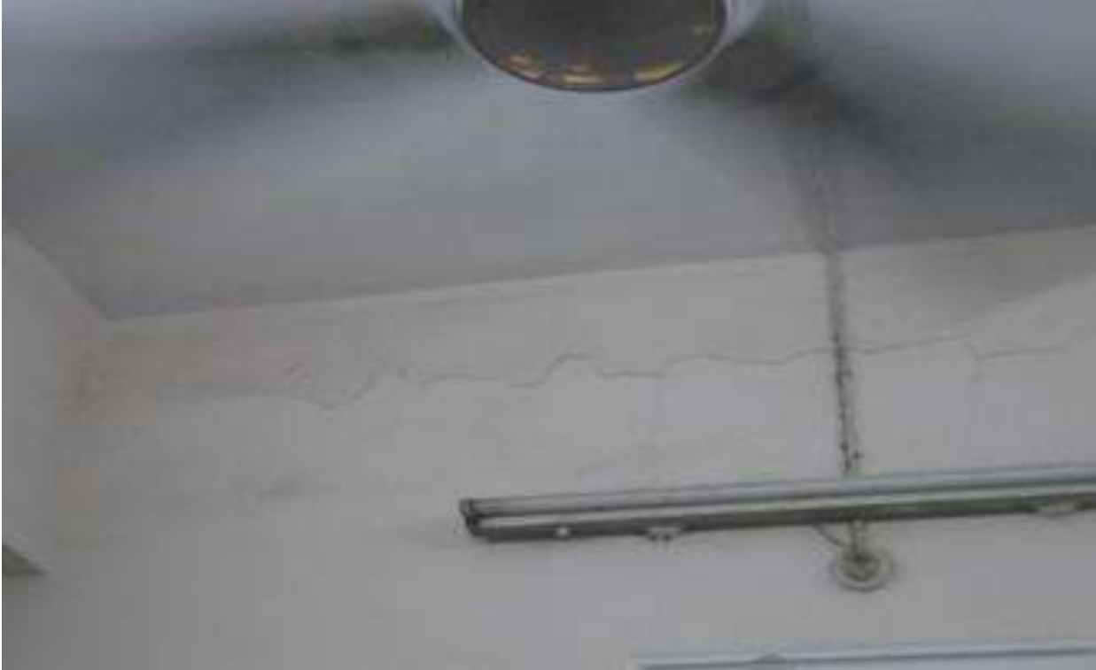
PH NO-10:-Photograph showing crack on beam at office no- 24.
