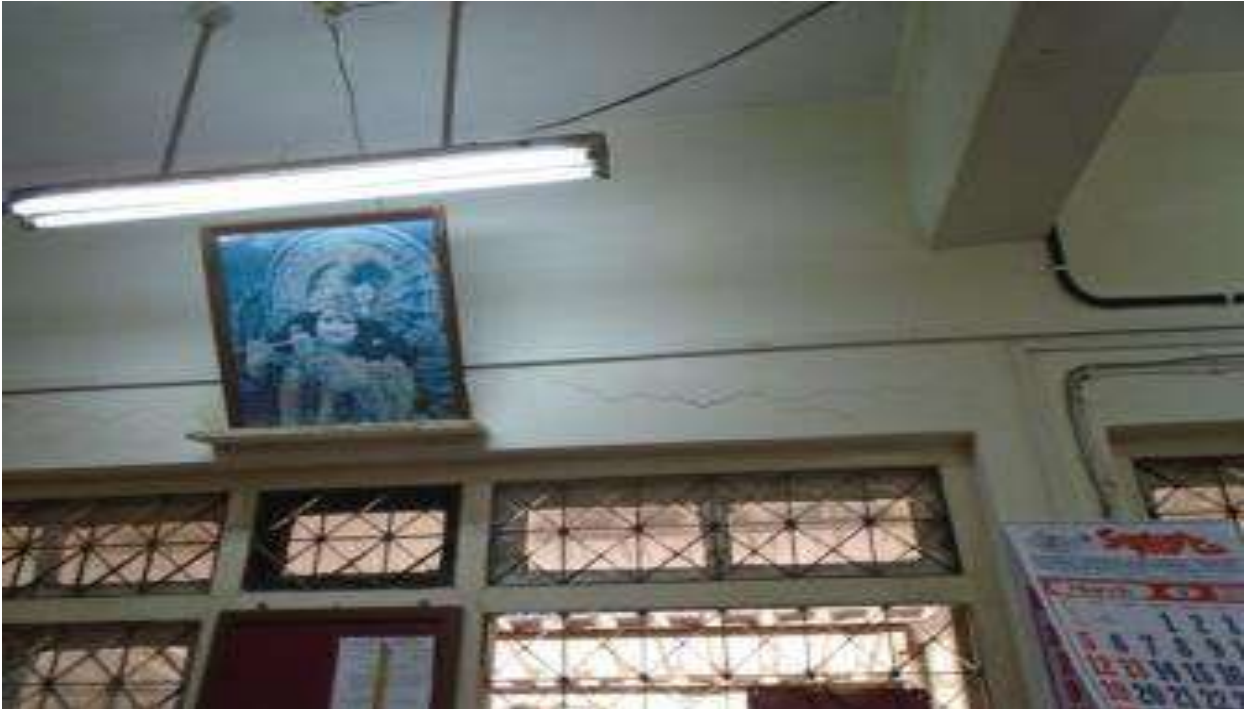
PH NO-22:-Photograph showing crack on lintel beam above window at office no-13.
