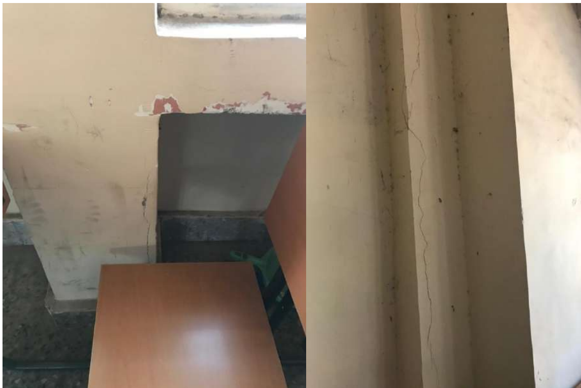
PH NO-43 & 44:-Photograph showing crack on column at various locations of room no-21.
