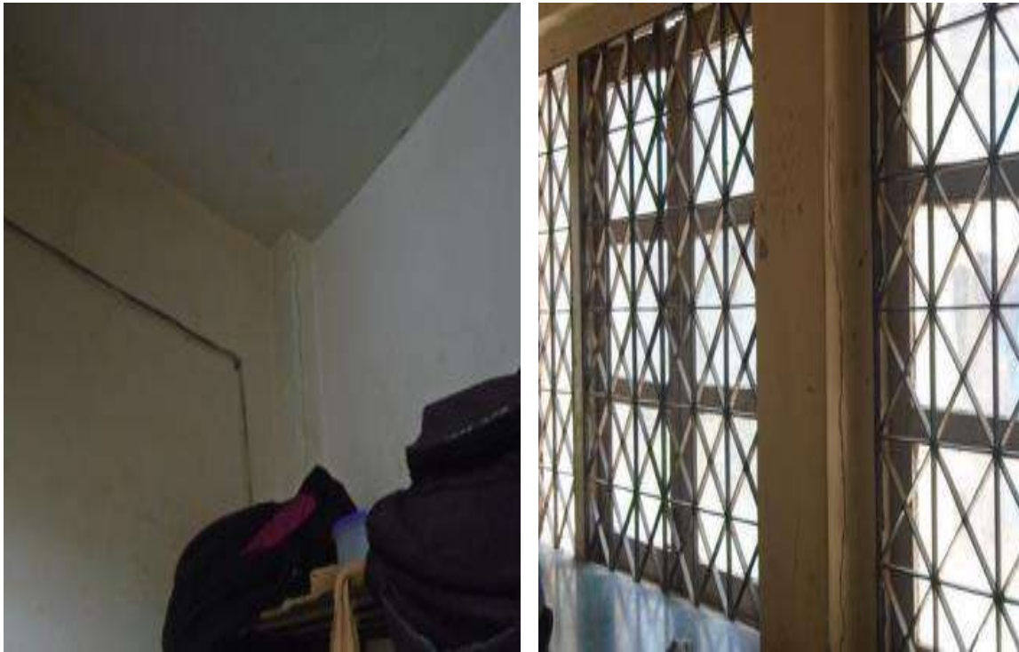
PH NO-35 & 36:-Photograph showing crack on column at various locations of canteen.
