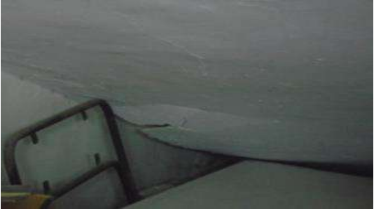
PH NO-33:-Photograph showing bulge of concrete cover on slab at store room.
