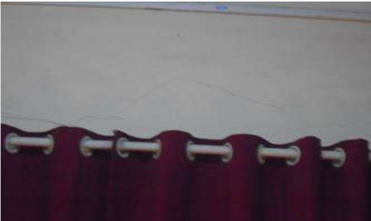
PH NO-32:-Photograph showing crack on beam at sports room.
