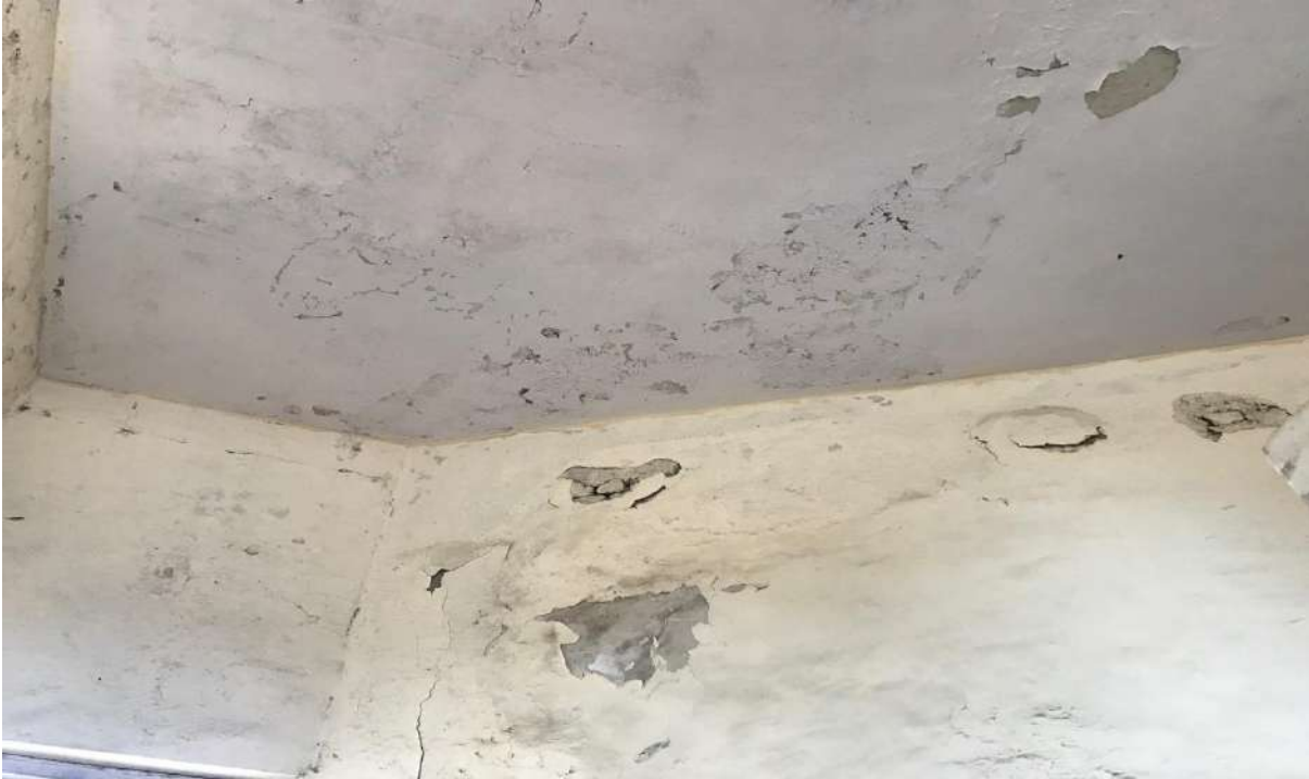
PH NO-51:-Photograph showing de bonded concrete cover on beam at second floor staircase area.
