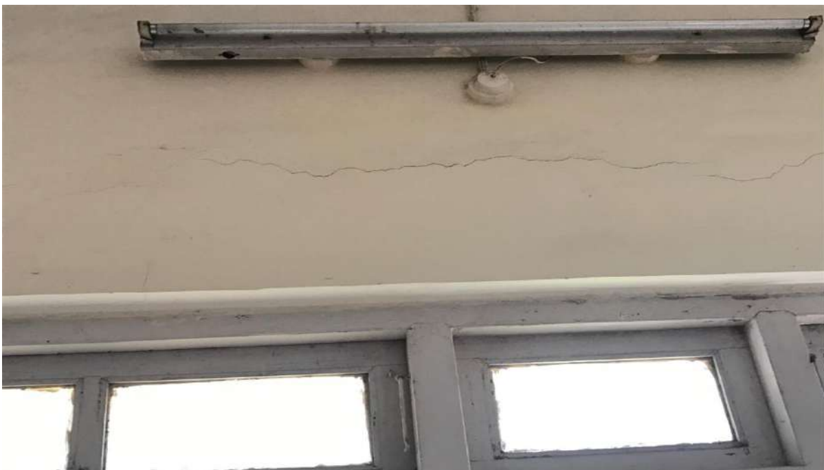
PH NO-46:-Photograph showing structural crack on lintel beam above window room no-17.
