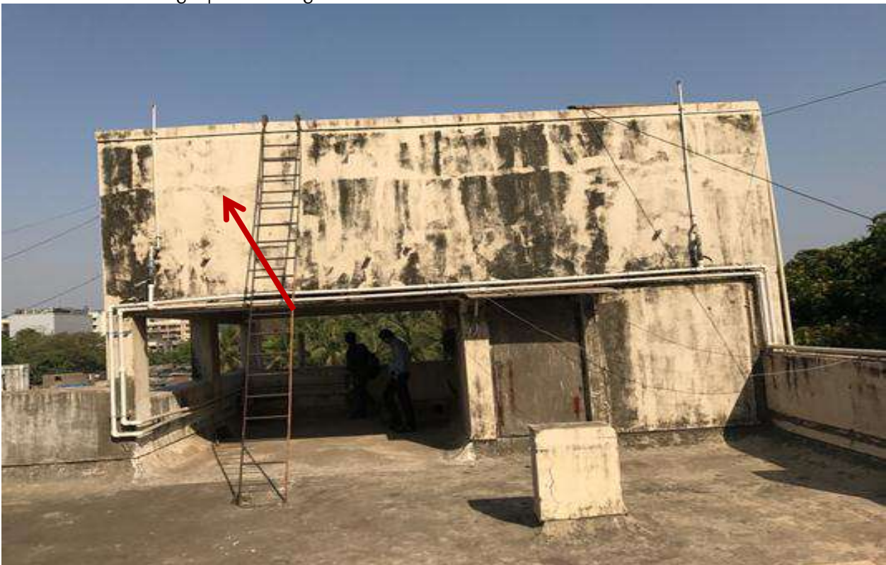
PH NO-23:-Photograph showing plaster crack on overhead tank wall.
