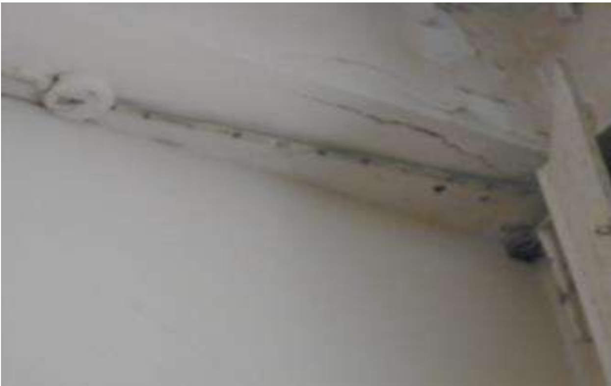
PH NO-09:-Photograph showing crack on beam.
