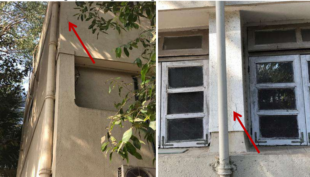
PH NO-10:-Photograph showing crack on column at various locations of existing structure.
