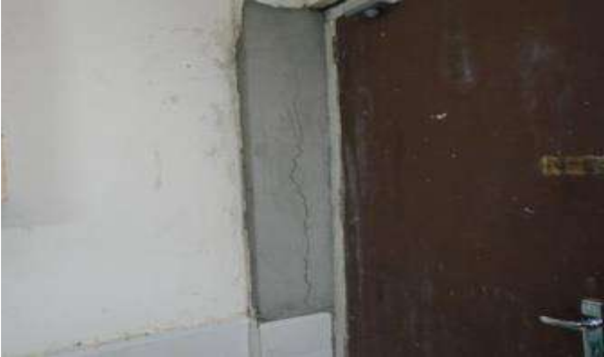
PH NO-14:-Photograph showing crack on column at office no- 32.
