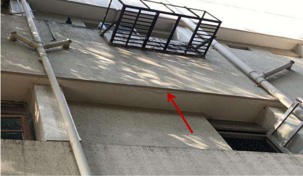
PH NO-11:-Photograph showing crack on beam. EAST
