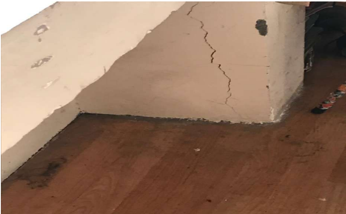
PH NO-48:-Photograph showing structural crack on column room no-14.
