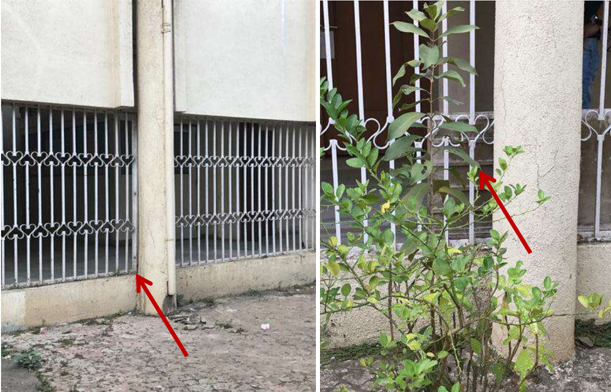
PH NO-14 & 15:-Photograph showing crack on circular column at various locations of existing structure.
