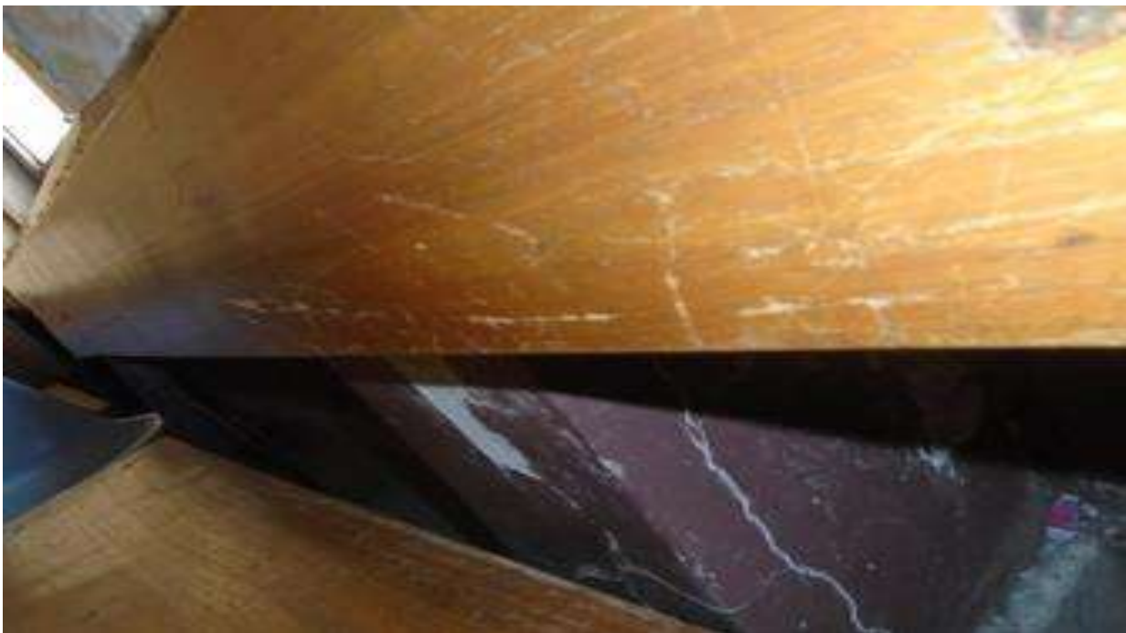
PH NO-37:-Photograph showing crack on column at various locations of room no-9.
