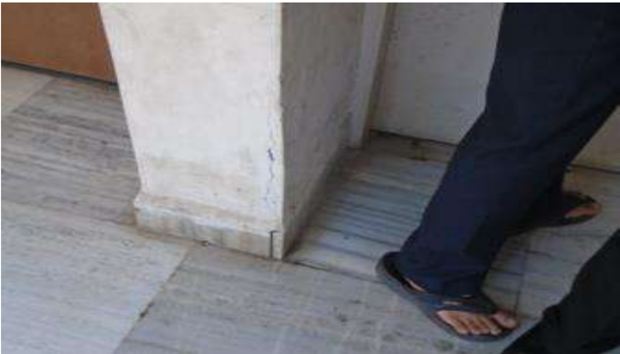
PH NO-20:-Photograph showing crack on column at various locations of passage.
