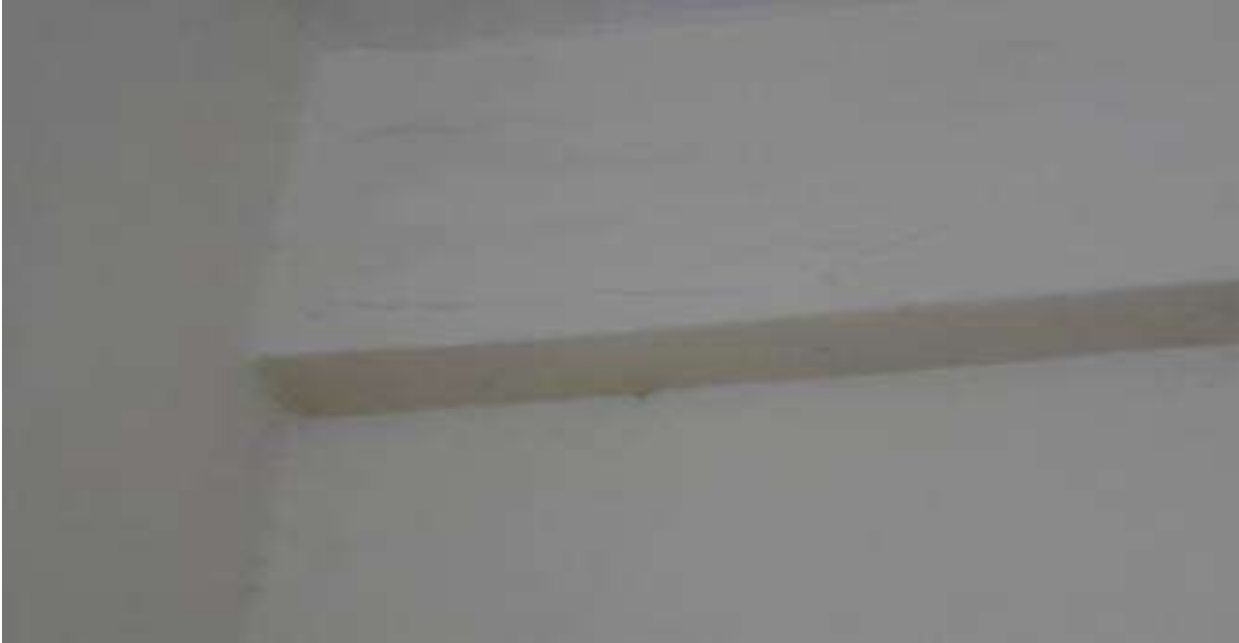
PH NO-12:-Photograph showing crack on beam at passage.
