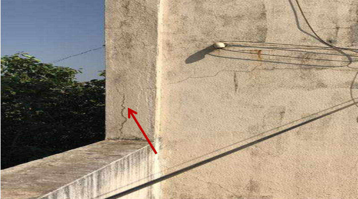
PH NO-22:-Photograph showing crack on column overhead tank .
