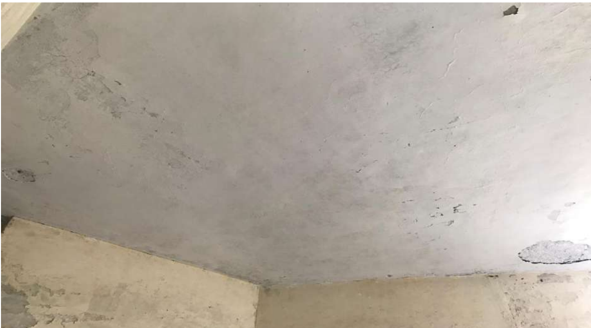
PH NO-52:-Photograph showing de bonded concrete cover on slab at second floor.
