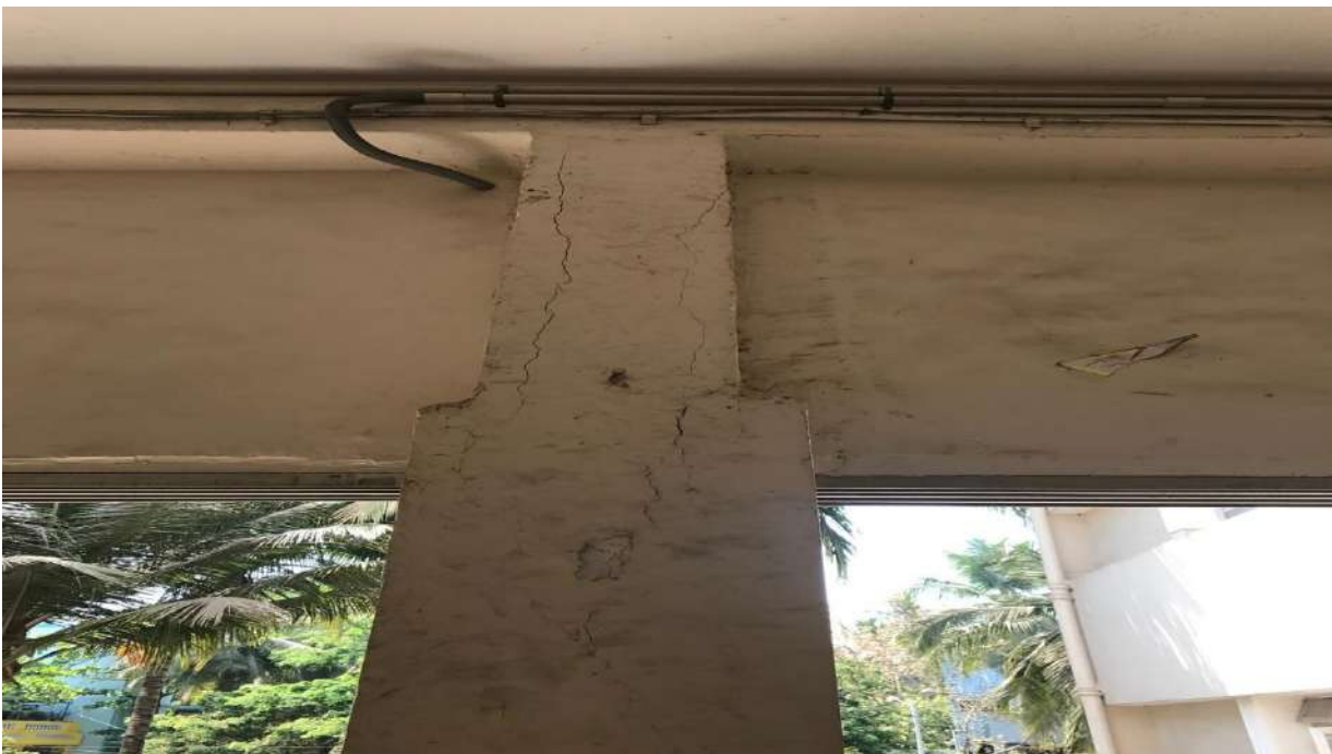
PH NO-39:-Photograph showing crack on column at some locations of passage.
