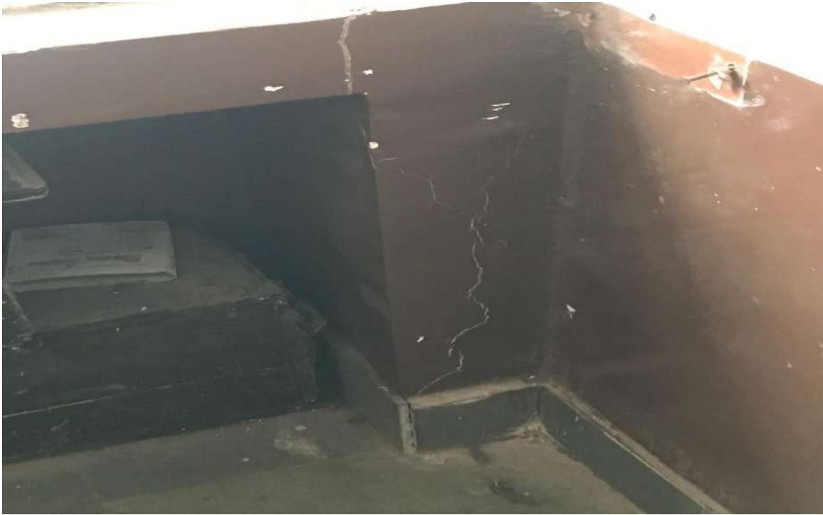
PH NO-49:-Photograph showing structural crack on column room no-15.
