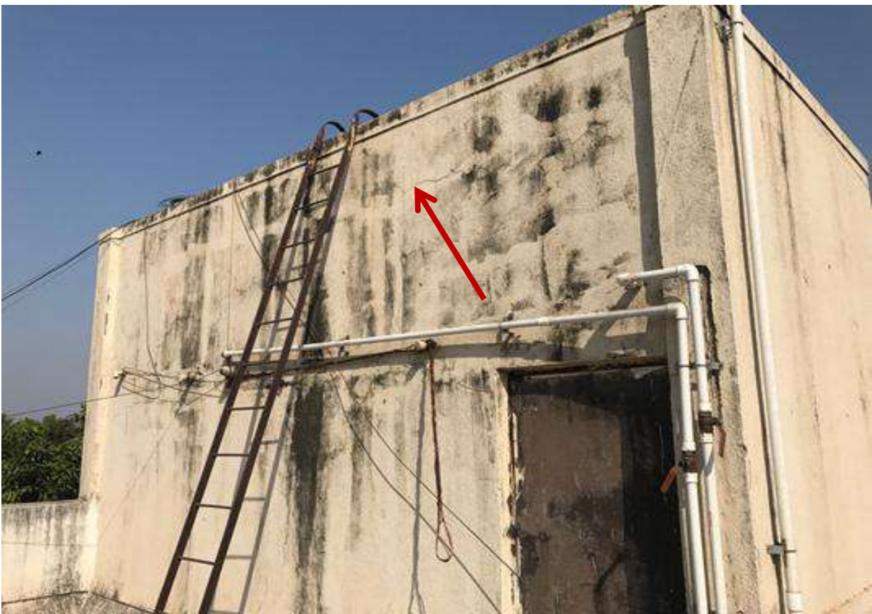
PH NO-22:-Photograph showing plaster crack on overhead tank wall.
