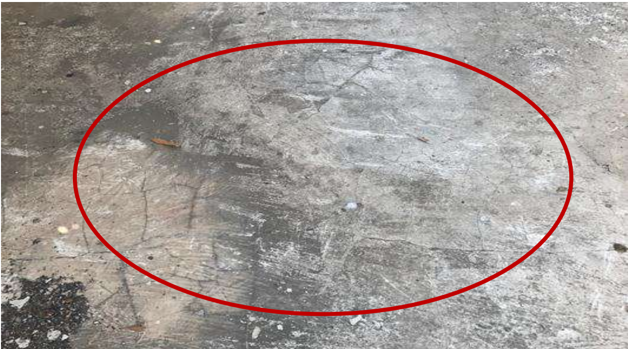
PH NO-20:-Photograph showing crack and de bonded concrete cover on IPS waterproofing.
