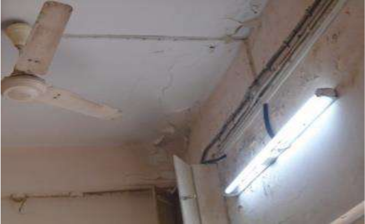
PH NO-07:-Photograph showing crack on slab.
