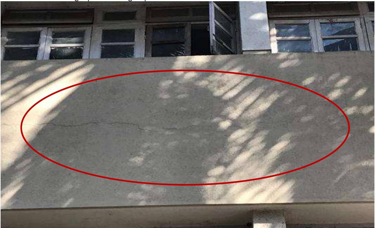
PH NO-05:-Photograph showing crack on RCC pardi at various locations.
