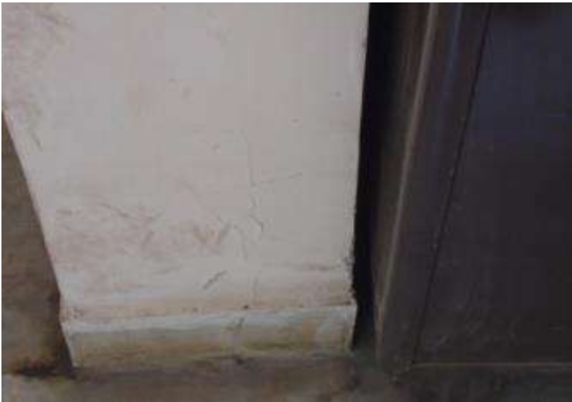
PH NO-26:-Photograph showing crack on column at passage.
