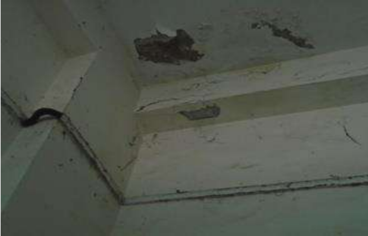
PH NO-38:-Photograph showing crack on beam at gents toilet.
