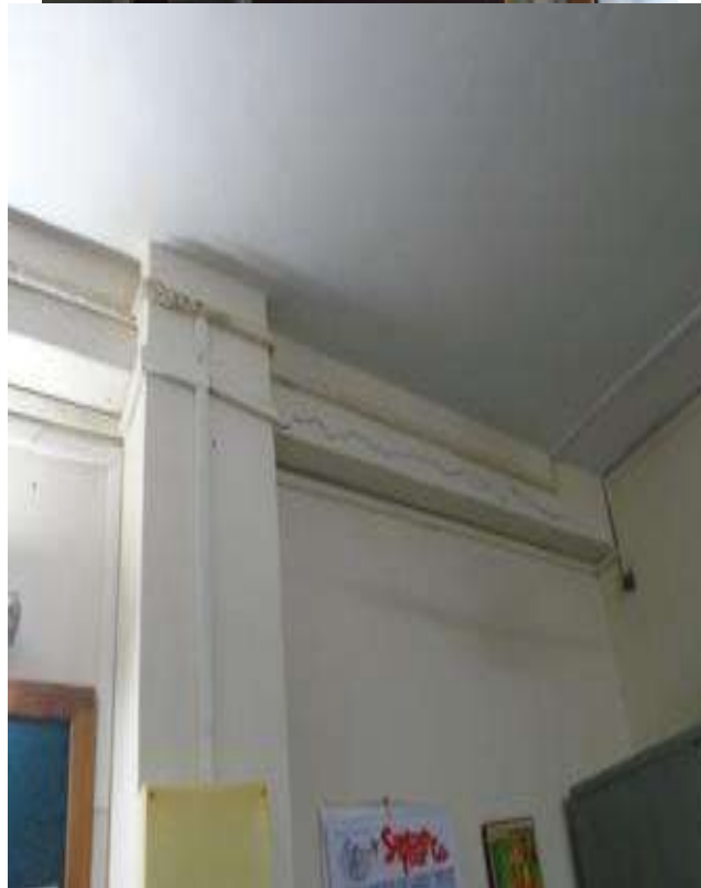
PH NO-15 & 16:-Photograph showing crack on beam at office no- 32.
