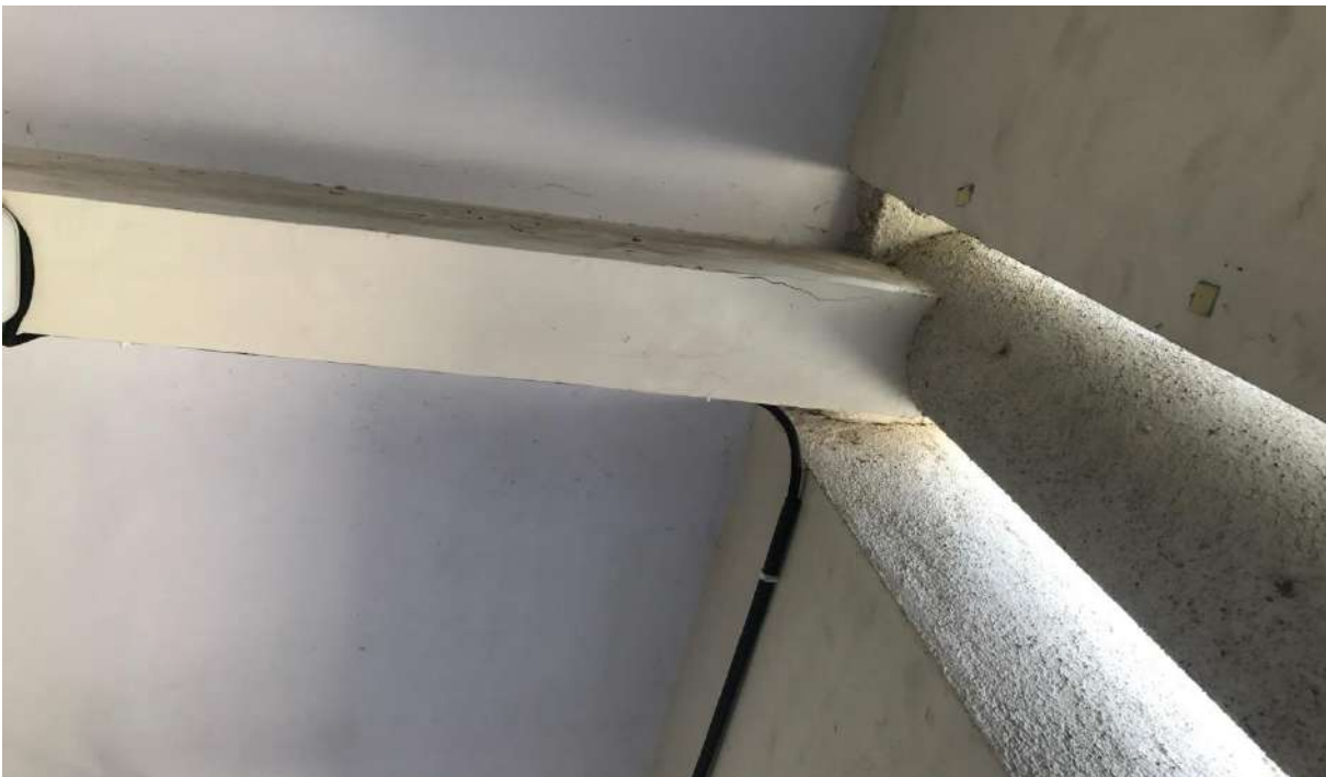
PH NO-41:-Photograph showing crack on beam at various locations of passage.
