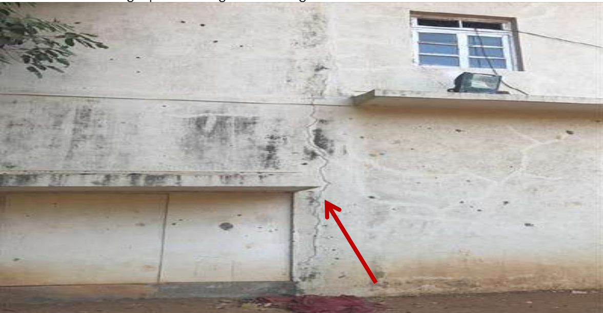
PH NO-19:-Photograph showing structural crack on column and surface crack on external wall in patches.
