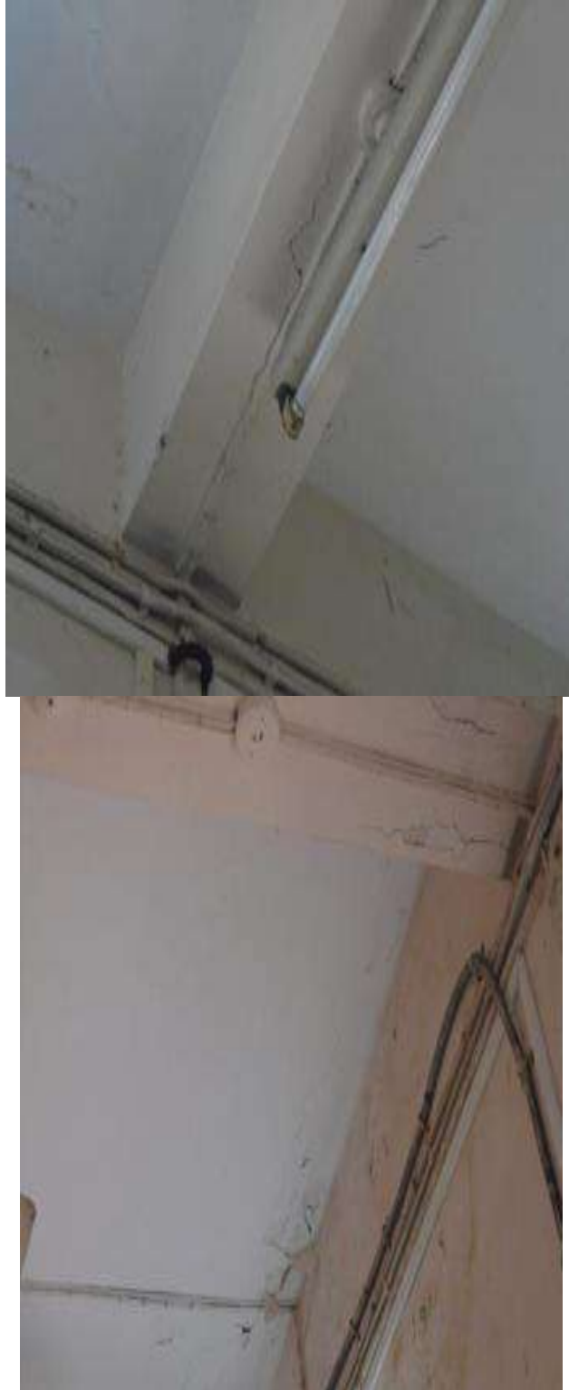
PH NO-05 & 06:-Photograph showing cracks on beam at office no -27.
