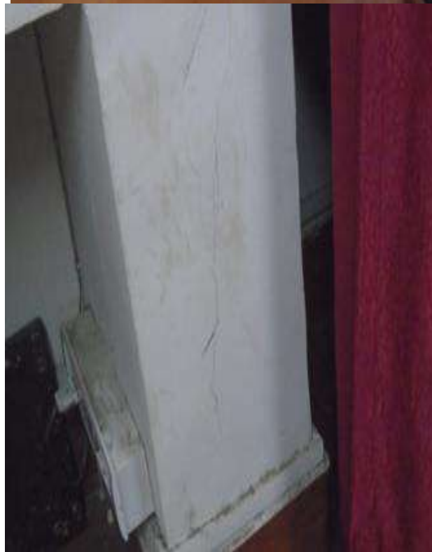
PH NO-29 & 30:-Photograph showing crack on column at various locations of auditorium.
