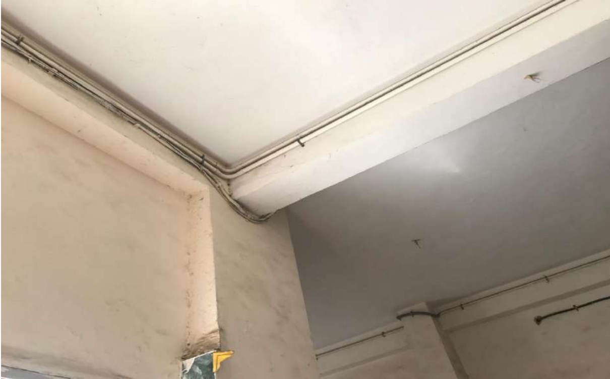
PH NO-40:-Photograph showing crack on beam at passage.
