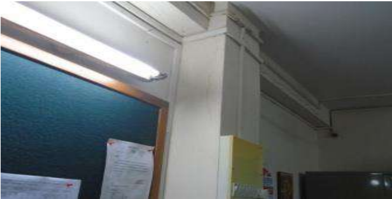
PH NO-18:-Photograph showing crack on column.
