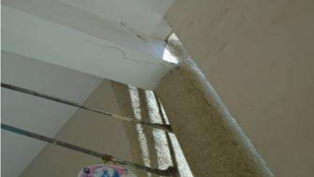
PH NO-19:-Photograph showing crack on column and beam at various locations of passage.
