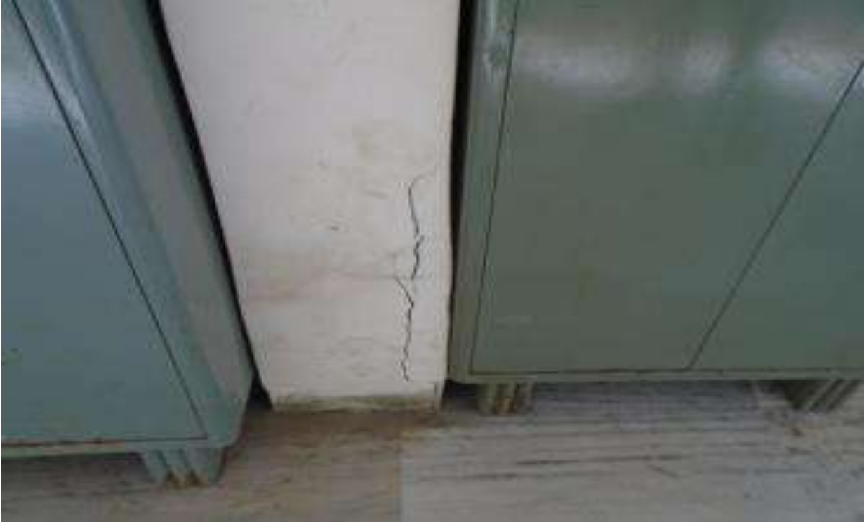
PH NO-23:-Photograph showing crack on column.
