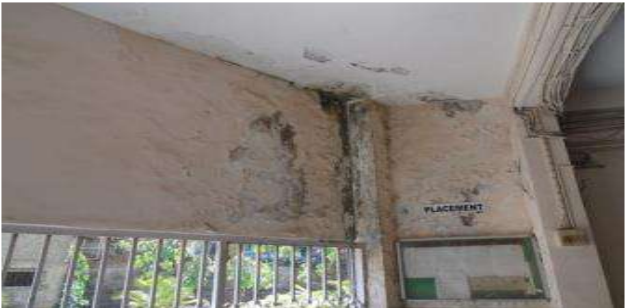
PH NO-28:-Photograph showing leakage mark on column and wall at passage.
