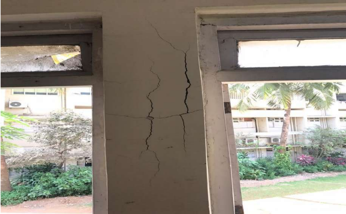
PH NO-45:-Photograph showing structural crack on column at various locations of room no-17.
