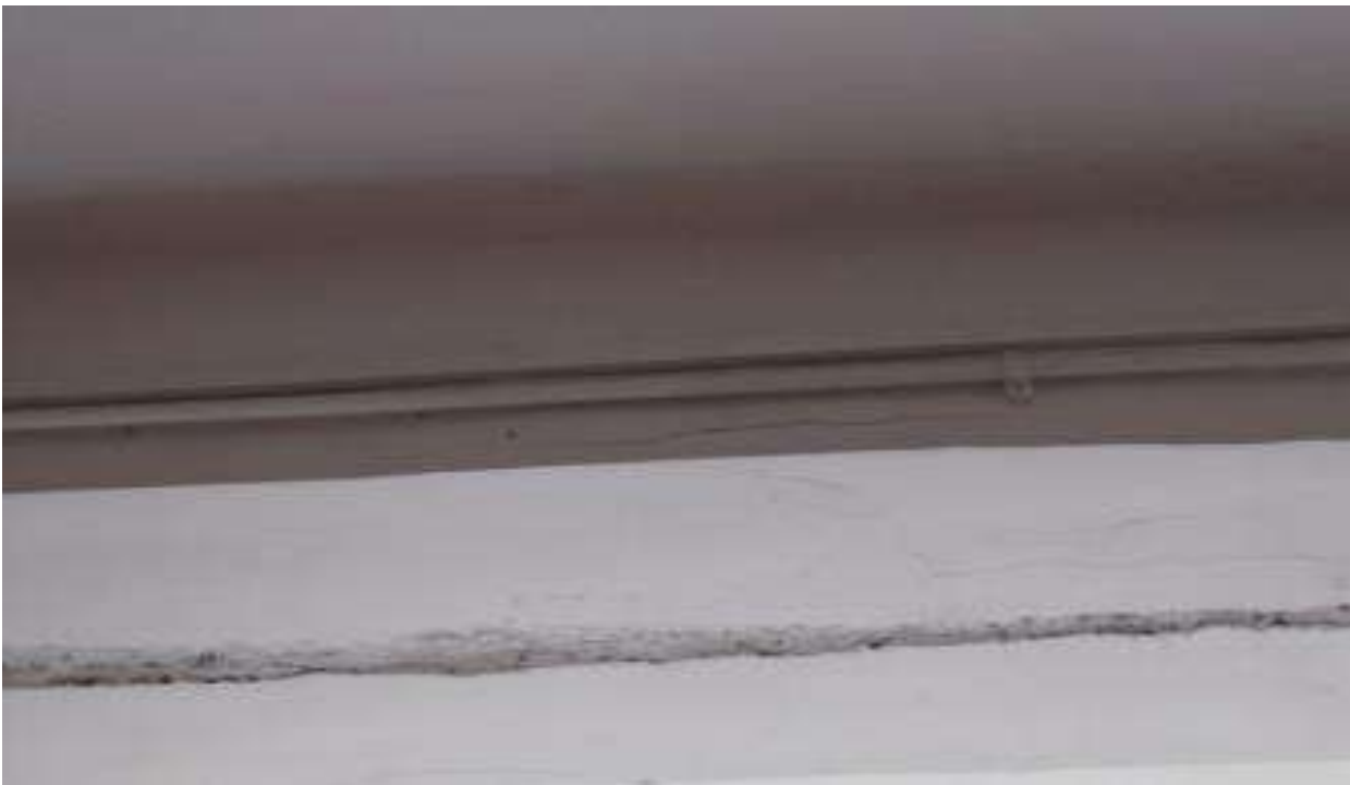
PH NO-13:-Photograph showing crack on beam at passage.
