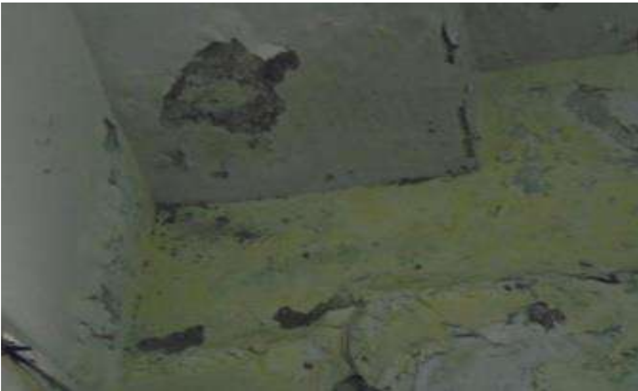
PH NO-34:-Photograph showing leakage mark and peeling of paint on sunken slab at gent's toilet.
