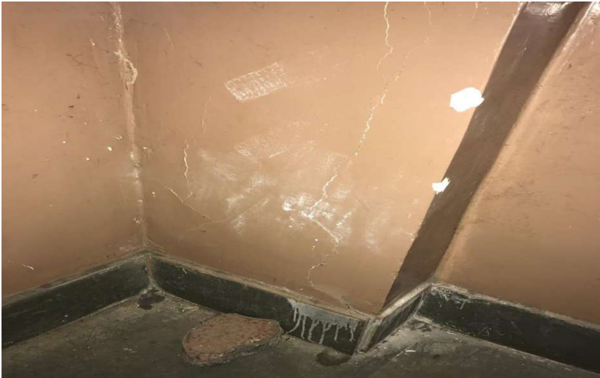
PH NO-47:-Photograph showing structural crack on column room no-16.
