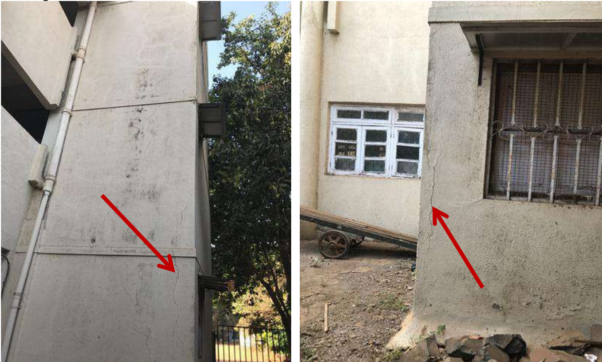
PH NO-16 & 17:-Photograph showing crack on column at various locations of existing structure
