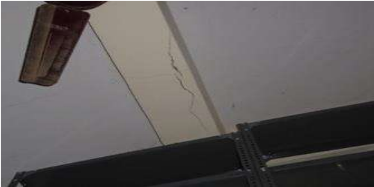
PH NO-01:-Photograph showing crack on beam bottom at staircase area.
